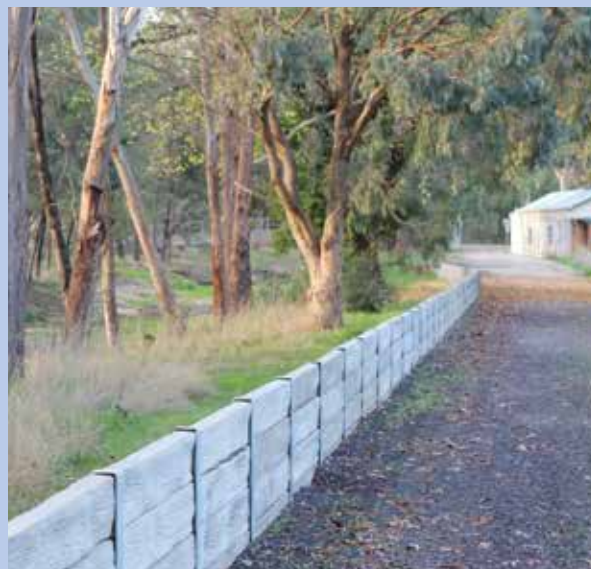
Levees can take different forms – this wall is designed to fit along a narrow strip of public land, and to look appealing for overlooking properties.
